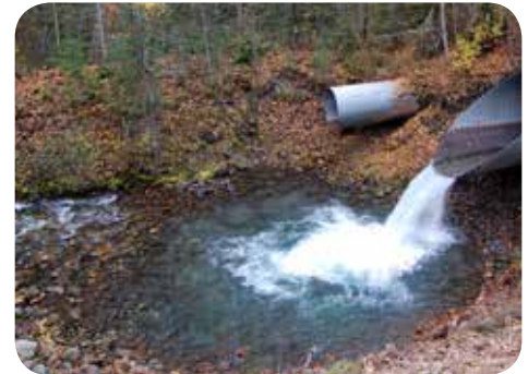
A perched culvert prevents upstream movement of most fish species. Photo: K. Maier, Gwich'in Renewable Resources Board
